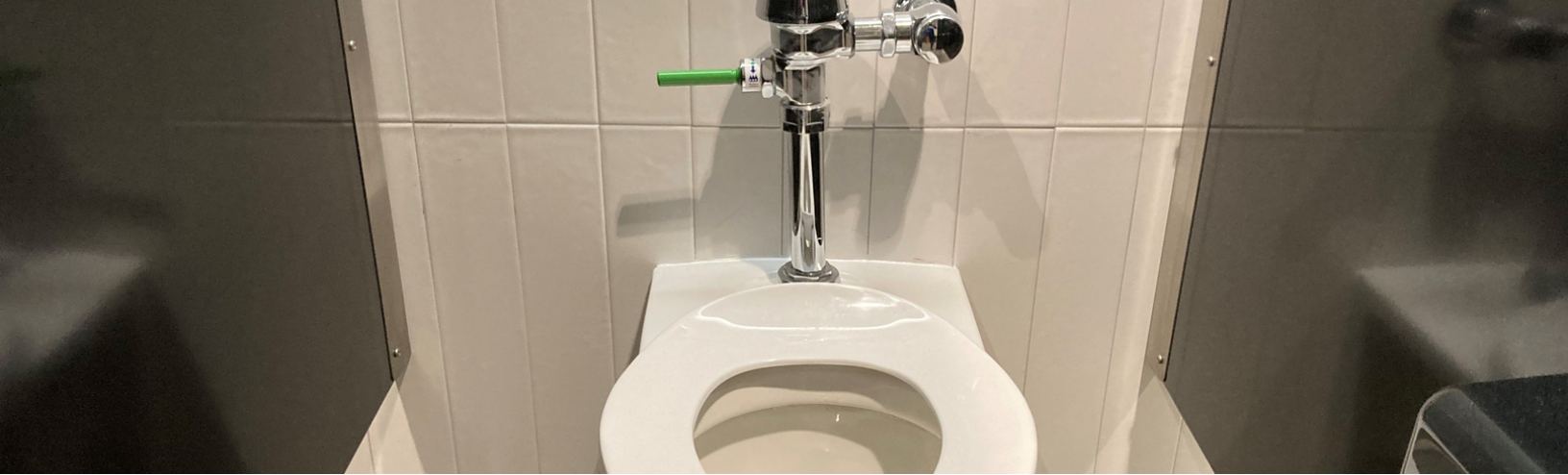
PHOTO 4: LOW FLOW FIXTURES
