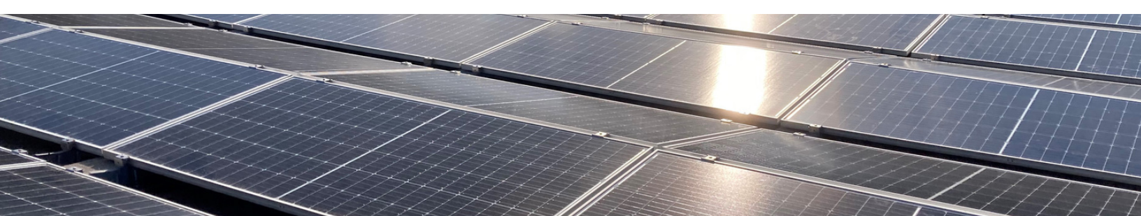
PHOTO 3. SOLAR PV ON ARTS CENTRE ADDITION
